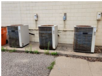
Existing Library Compressors
